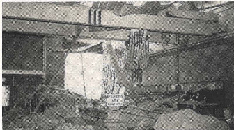
Brick and tile blown out by the explosion fell through the roof of the maintenance shop, shown here, and other parts of the office section. The debris has been removed and work is underway on repairing the damage.
