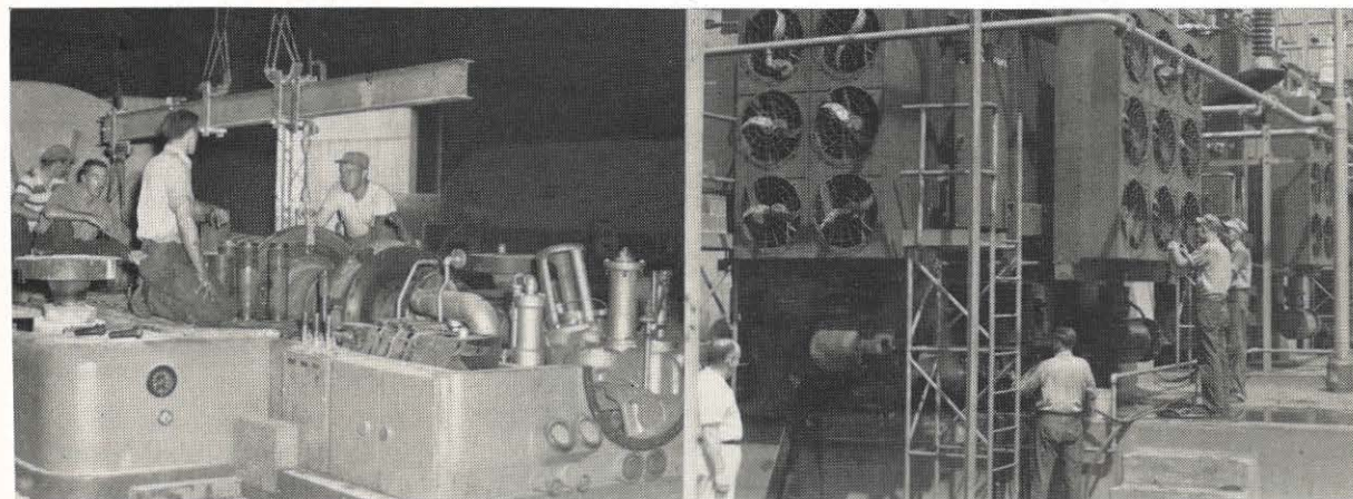
The last of the four units at Philip Sporn plant was scheduled to return to service August 1 after a general overhaul. The other three units have been off at various times since the first of the year, usually four weeks at a time, for similar work. The last one, Unit 3, was taken off June 30. LEFT: Four employees dismantle the high pressure turbine. From the left they are George Bush, helper; Charles Yeager, master maintenance man; Homer Gordon, master maintenance man; and James Bearhs, helper.
