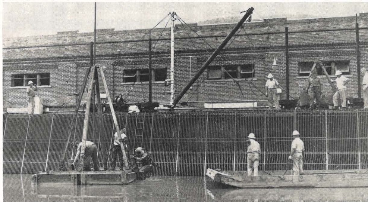
Roy Easter descends into the water at Byllesby hydro to fasten a cable around a log lodged in the mud against the trash rack bars. In the left foreground is the pontoon used for supporting the jetting nozzles and in center is a stiff-leg boom to carry the hoist cable. The two men at the right are standing in a barge used to haul away trash and debris.
