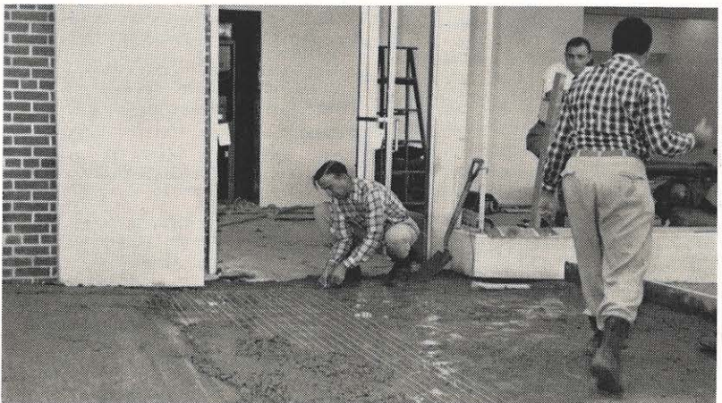
There'll be no slipping and sliding from snow in front of the new Pearisburg office building of the Bluefield district. Electric heating cable, contributed by a manufacturer, has been installed under the concrete sidewalk. Here, John B. Kahle, left, and Archie Phlegar, with back to camera at right, are installing the cable as James R. Boulton, area sales representative, looks on. Mr. Kahle and Mr. Phlegar are heating and builder sales representatives. The 1600-watt cable is 582 feet long and covers an area of about 120 square feet.
