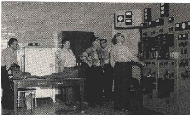
Appalachian system employees cut in the first circuit from Philip Sporn plant to Kaiser Aluminum and Chemical Corporation's substation at Willow Grove. Shown above are from left: A. B. Purdy, system relay; Ken Martin, system meter; Kermit Ford, system substation operator; R. B. Greer, system relay, and L. B. Ferguson, system substation supervisor, who is throwing the switch. This line is the first of four that are planned to operate at 132,000 volts to supply power to the huge Kaiser plant. Ohio Power will supply the power through Sporn plant. The new line replaces a temporary 33 kv line. The Kaiser station was energized November 2.
