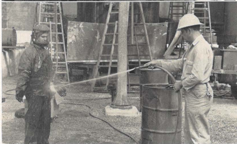
TOP: Two members of the transformer maintenance crew remove old paint from a 132 kv transformer with a hot caustic application. The caustic is heated in the mobile tank in the foreground and pumped through the hose to the top of the transformer where it is flowed over the surface, stripping the paint off down to the bare metal. This comes after gasketing and is followed by painting. BOTTOM: L. B. Heptinstall, left, has just come off a transformer after applying hot caustic. As a safety measure he is being washed down—to get all caustic off—by J. E. Glover. Caustic work calls for the men to wear rubber suits, masks, helmets, gloves and protective boots.
