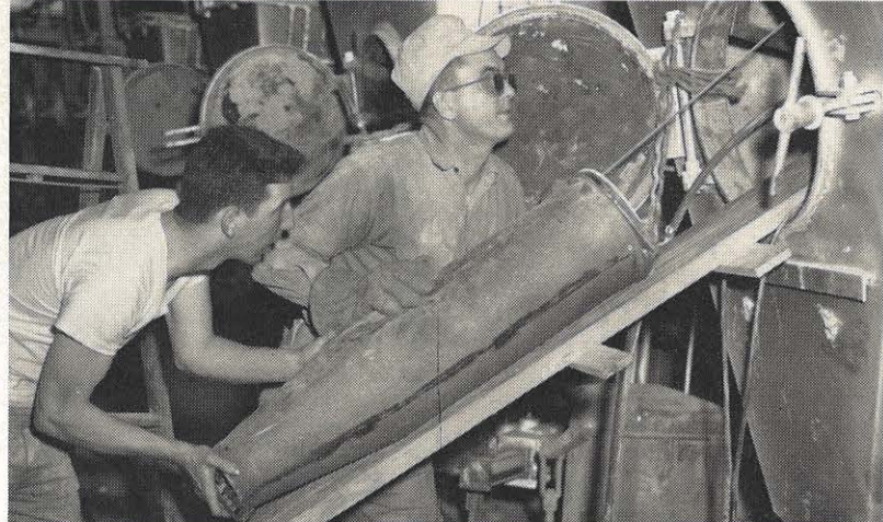
At the other end, F. D. Carelli and S. E. Kees have pulled the lifting cable through the side of the boiler hopper and down through the new tube. Note the hook at the lower end of the tube. They are assisting in getting the tube back up into the hopper, pushing as the lifting cable is being pulled from the other end.
