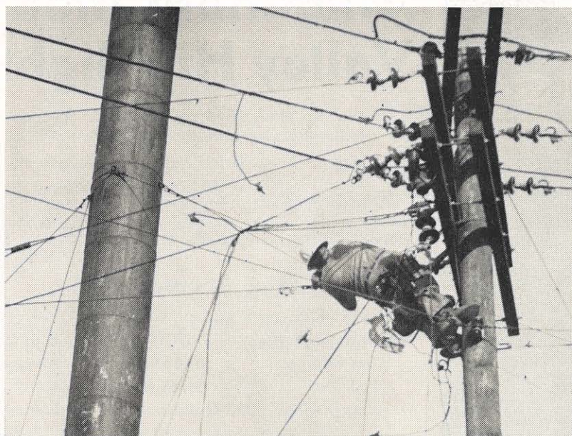
C. T. Rader, Roanoke lineman, is repairing four 4,000 volt lines and two street light wires which were broken when a cupola was blown from a building, tearing the lines in its decent to the street. Photo courtesy 'Roanoke World-News.'
