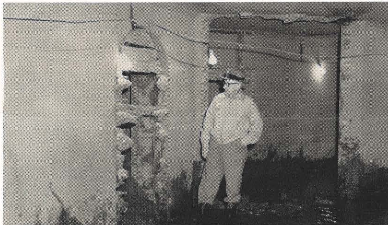
L. E. Turner, Glen Lyn plant manager, was photographed recently at the same spot in the plant tunnel where a similar picture was made in 1923. He was the last one out of the tunnel that year before water was allowed in. The tunnel had been in continuous use until recently.
