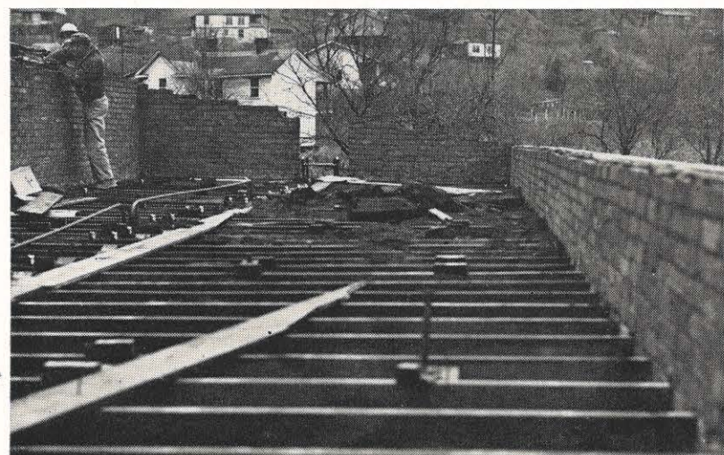
This is one section of the top of the garage and storage building at Lothair that was destroyed by a wind storm. The roof was lifted off and hurled to a nearby railroad track. John K. Cody, Hazard substation, is examining the damage.
