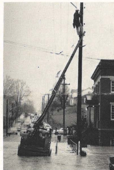
Clyde E. Wysor, meter serviceman, disconnects service to a church ahead of the rising flood waters in Bluefield, Virginia. This and other preventive measures were undertaken throughout the area in the short time before the floods.
