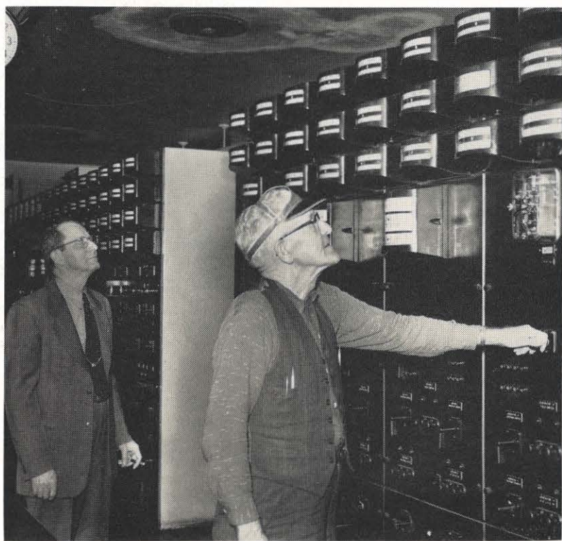
Checking current on Generator A at Logan plant after the plant returned to service March 8 are C. E. Marshall, dispatcher at left, and Sam Woody, control operator. The plant has been off the line since the flood on January 29. During the work, 81 electrical motors that had been submerged were overhauled and all operating equipment checked and cleaned. Two shifts of 10 hours each, composed of both maintenance men and operators, worked as units to repair the damage from the worst flood in Logan's history. The plant's safety record was kept intact through the repair period.
