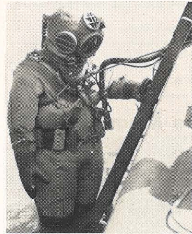
Descending into the river, a diver prepares to cut the cells and connecting wall, by means of a cutting electrode, below river level. Some of the cells and part of the connecting wall were cut off ten feet below the river surface in order to permit water to enter the screen house. Normal depth of the water at the screen house is 24 feet.
