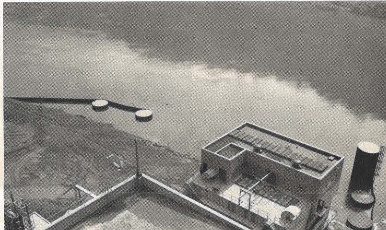
The completed diversion wall is almost invisible after the cells have been cut off, filled with sand and gravel and capped with concrete. Only five of the eight cells can be seen above water, but all are working to let water in while keeping debris out.
