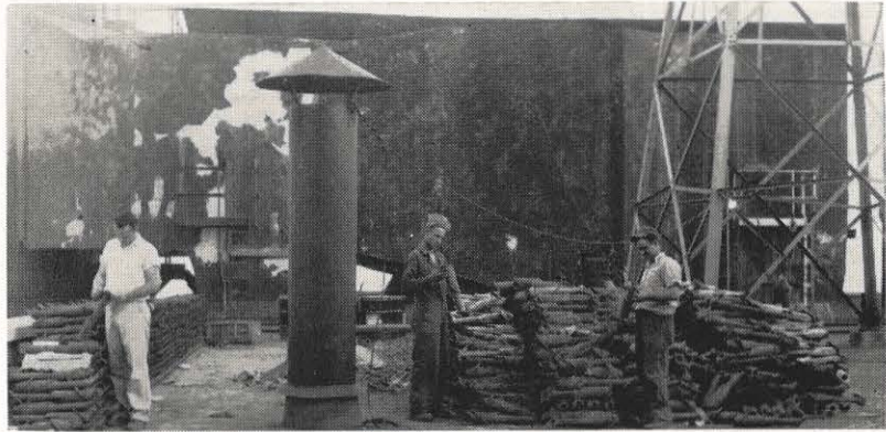
Shown at work during the outage of Philip Sporn plant Unit No. 1 are three plant employees. From left: William Soulsby, maintenance helper, inspects new tubes for the dust collector, while Paul Fitzgerald, maintenance man, and Fred Smith, laborer, inspect the worn tubes. In the background is the dust collector housing in which the new tubes will be placed.
