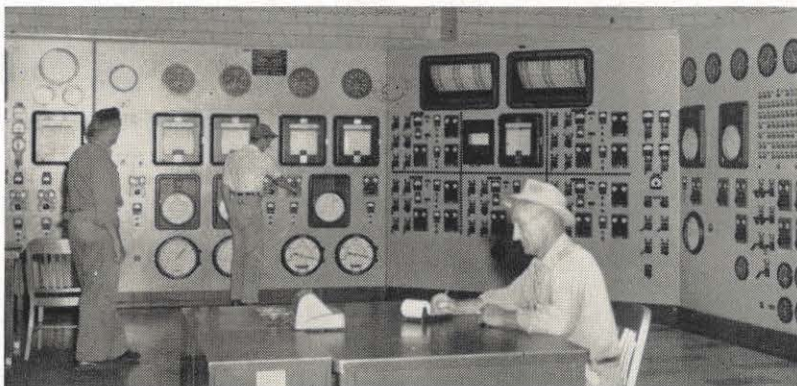
Demand for electricity slacks off at night when the majority of our customers are asleep. Here, at Philip Sporn plant, these employees in the control room are reducing the load on the units for this night curtailment. They are from left: William Wentzell, control operator; D. A. Cadle, auxiliary equipment operator; and Clarence Tennant, shift operating engineer.
