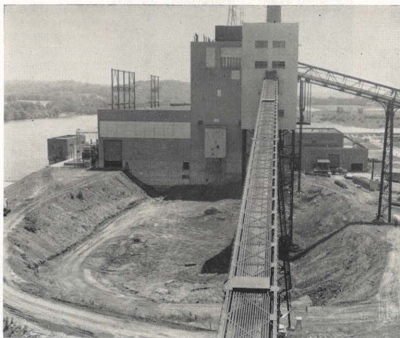
Excavation has begun for the new 450,000 kw unit of Philip Sporn plant.
