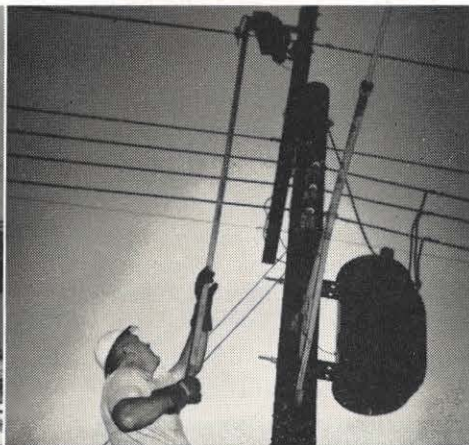
Serviceman E. A. Berginnis locates the trouble spot and prepares to climb a pole to restore service. He has talked with the dispatcher and with line supervisor W. E. Mitchell, who gives him additional information about the locality, and has put on his safety and climbing gear. At this point he plans the job ahead. RIGHT: On the pole Mr. Berginnis, with the night sky a backdrop, opens the cut-out housing with his switch stick and replaces a fuse. Lights go on in the nearby house and another night emergency job is completed.
