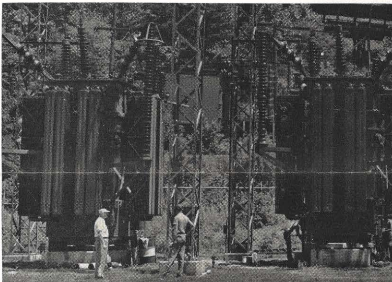
The Hazard switchyard is back in full operation. A 45,000 kva transformer, damaged in the flood January 29, has been returned to service after repairs by Westinghouse. Shown inspecting the transformer are Gaine Stidham, Hazard district superintendent, and Tom Old, system station. At right is another of the three transformers that make up the switchyard's 135,000 kva bank. Between the two, in the background, is a 15,000 kva mobile unit that was used while the damaged transformer was away for repairs.
