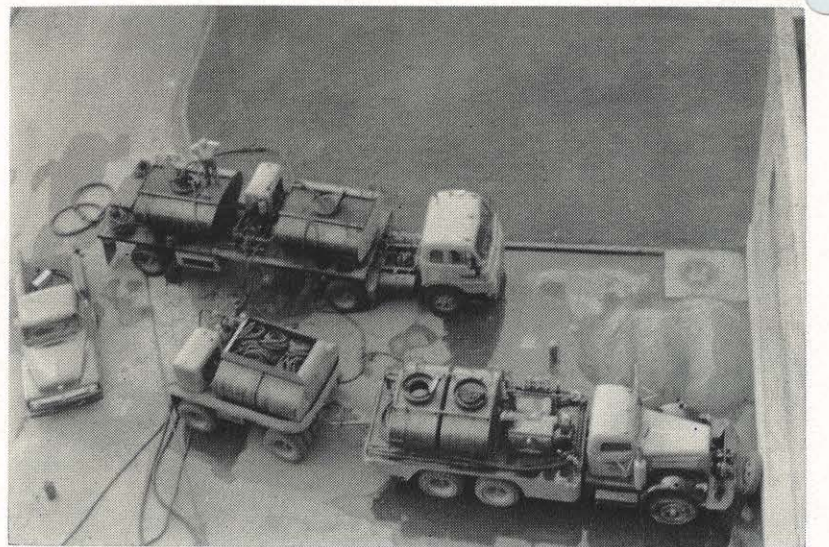
This equipment was necessary when the boiler of Unit No. 4 at Philip Sporn plant was given a recent acid bath. In addition to the trucks shown, a rail-road tank car holding the acid took part in the operation. The unit was taken out of service June 27 and returned July 15 after an overhaul. Dust collector tubes were replaced and control and intercept valves were cleaned. The boiler was washed with acid for the first time since it was put in service. This bath was to remove any scale or deposits that might have accumulated in the boiler tubes and drum.
