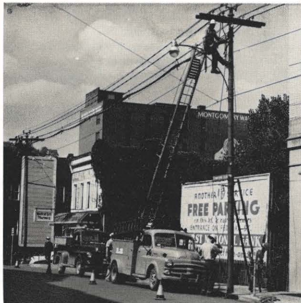
The before and after of the Bluefield business section distribution system is shown in these pictures. At left, employees begin removing 4,000-volt circuits. At right the new 12,000-volt aerial cable has been installed. The "after" picture, taken at a slightly different angle, shows
