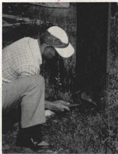
D. R. Spicer, line and station employee, inspects one of 65,000 poles in the Roanoke district. These poles are currently being checked under a pole inspection program. In addition to making a record of all rotten or defective poles, inspectors note other corrections on the poles and their lines that should be made. The principal hazards in the district-wide check, according to Mr. Spicer, are dogs and poison ivy.
