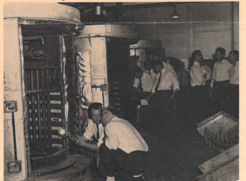
Test equipment, installed in the Philip Sporn plant in 1956, is examined by members of the ASME research committee. Kneeling in the foreground are Lyle Schueler of Diamond Power Specialty Corporation (left) and Philip Sporn plant manager A. G. Mehlman. In the background are representatives from our company, AGE and several other industries.
