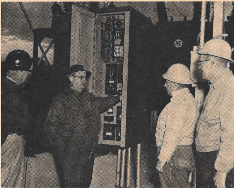
John Armstrong, system operating supervisor, switches Kingsport's new Orebank station into operation. Present when the 132/12 kv station went into service were from left: R. L. Herr, chief operator, Holston station; Mr. Armstrong; R. E. Wells, Kingsport station man and F. S. Russell, Kingsport line foreman.
