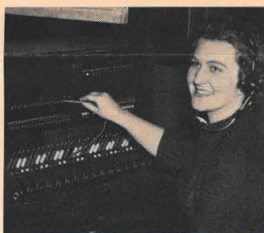
Patricia Dudley, Williamson district accounting department, demonstrates the district office's recently installed PBX, cord-type switchboard. In addition to other key communication points, this will permit dial communication between the service building on the Kentucky side of the river and the office in Williamson for the first time. Also, the system will improve answering service for customers in case of trouble.
