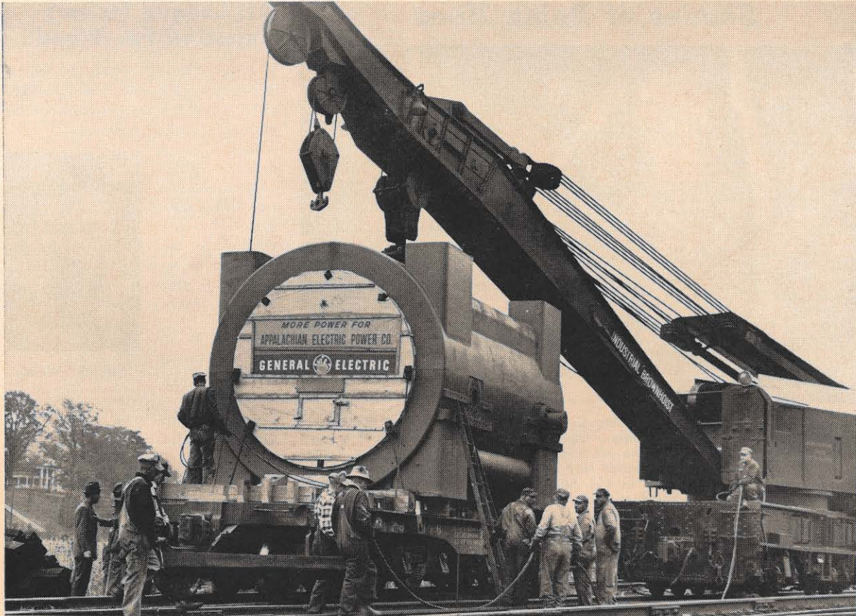
Norfolk and Western railroad workers secure the low pressure stator at Roanoke after transferring it by locomotive crane to another special low-bed flat car. The stator, shipped by General Electric from Schenectady, New York, is one of the two recently received for Clinch River Plant's number one generating unit.
