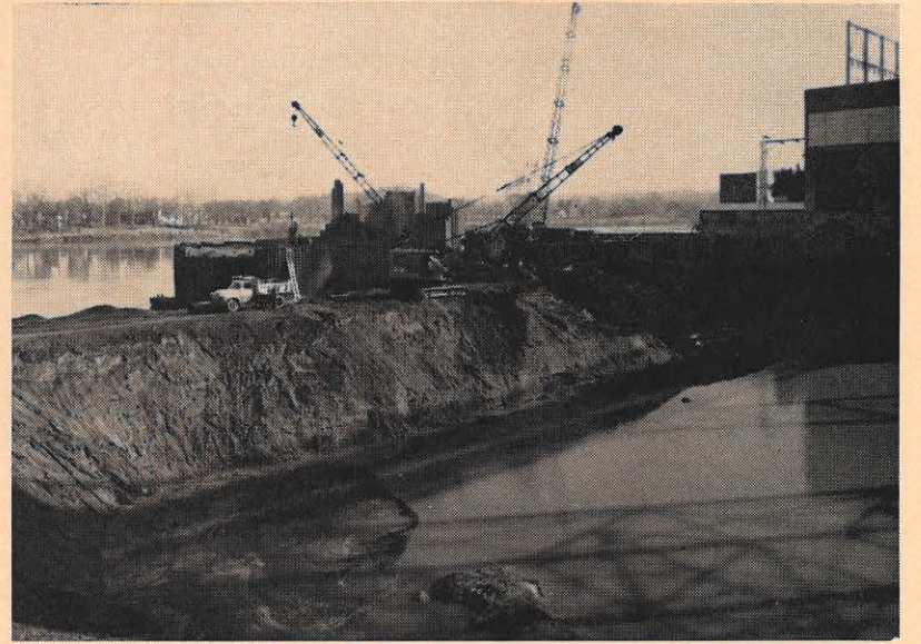
Pile driving in progress at Philip Sporn plant is shown in the center of this photo. This work, and the excavation in the foreground, are in preparation for the construction of a new 450,000 kw unit at the plant. A section of the plant is at right.
