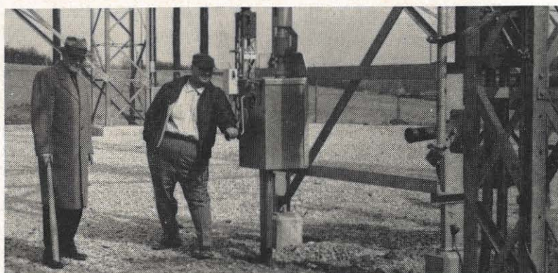
John Armstrong, right, throws the switch to energize the new 10,000-kva transformer recently installed in Pulaski district's 132-kv Floyd station. At left, Bruce Cox, Fieldale district manager, watches the operation which resulted in giving the Stuart-Woolwine area two sources of power.
