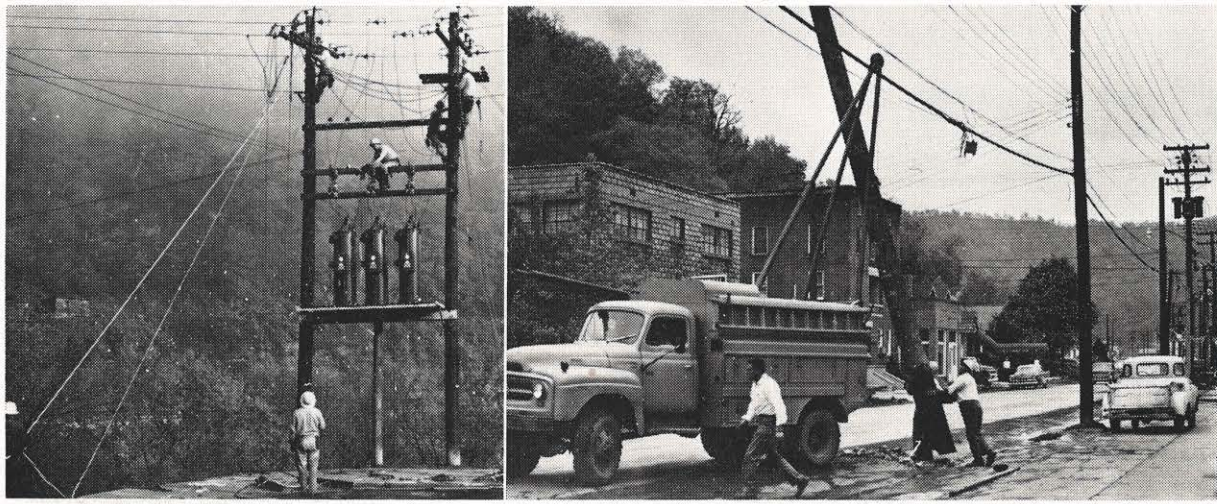
In the early morning hours, Kentucky Power Company employees (left) work on the 300 ampere regulator bank installed on the Blue Grass 4-kv circuit serving part of Hazard's business district. At right, workmen remove a
