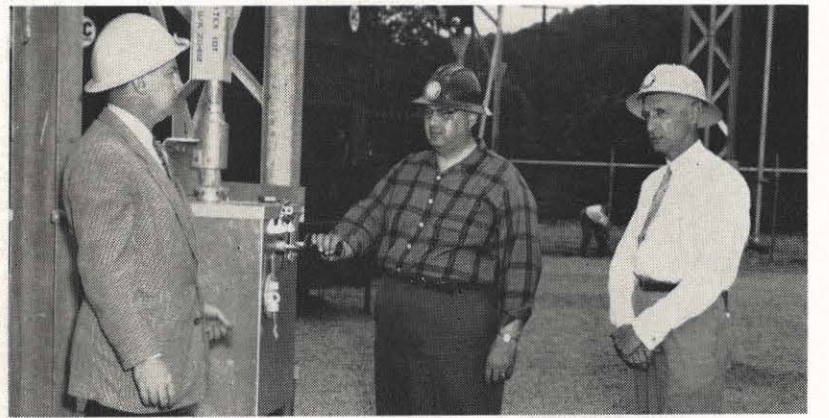
John J. Armstrong, center, system operating supervisor, throws the switch putting the new Kumis 138/12-kv station into service. At left is R. A. Armistead, Roanoke line and station supervisor. W. W. Krebs, Roanoke district superintendent, looks on at right.
