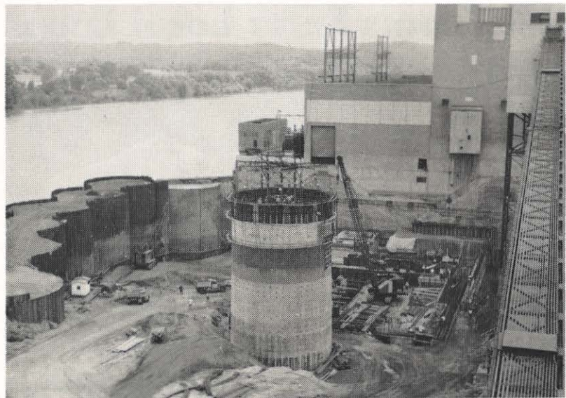
Beginning to rise from the excavation site of the new 450,000-kw unit at Philip Sporn plant is the stack, which will eventually be 602 feet high. Between the stack and plant are the boiler room area, turbine room area and heater bay area, where concrete pouring is underway. On the left are the temporary steel piling cells which hold out the river during construction, and on the right is the coal conveyor which transports coal to the plant.
