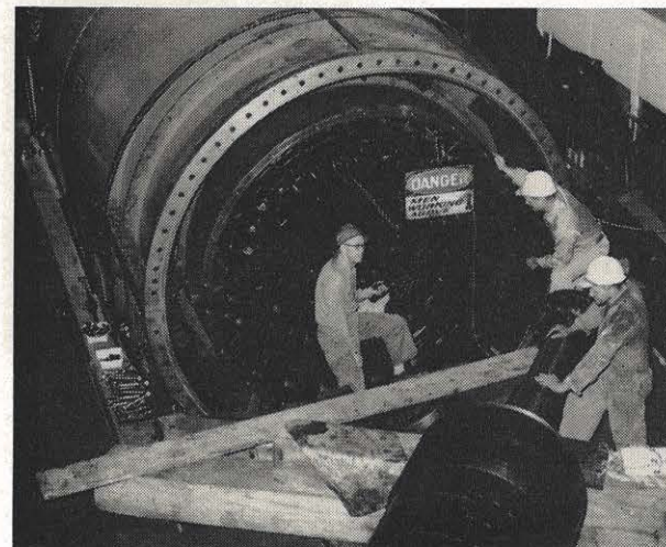
The annual maintenance overhaul at Logan plant has been completed. This year it consisted mainly of repairs to boiler A and Unit A, although the entire plant was down for a period for inspection. At left, C. H. Feiszli, G. W. McAbee and W. C. Blankenship are inspecting the stator of Unit A. Work on this unit consisted of removing
