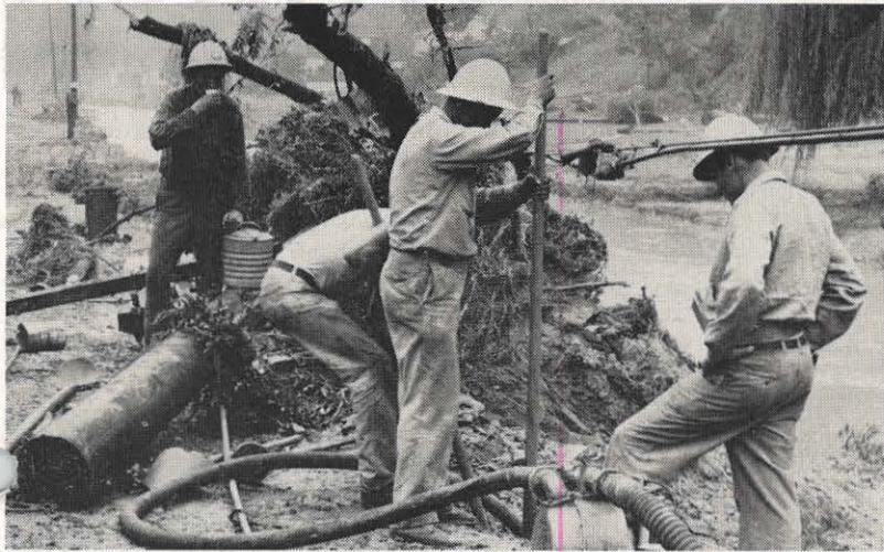
Lines were down and other company facilities hit when a flash flood struck in the vicinity of Charleston August 8. Here, Charleston employees work under emergency conditions to speedily restore service to the area. Picture courtesy "Charleston Daily Mail."
