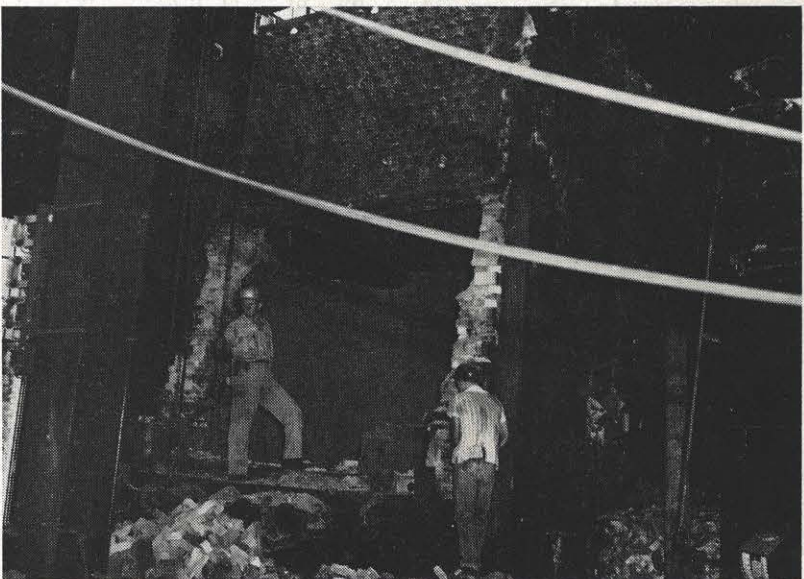
Boiler No. 7 of the old Hazard steam plant is dismantled by workers of Platnick Brothers Scrap Iron and Metals Company of Bluefield. The stack and most of the equipment will be removed from the plant which was retired recently after over 40 years' service. A large portion of the building will remain intact to house control equipment for the Hazard station. The plant, on stand-by status since 1954, had a generating capacity of 13,000-kw.
