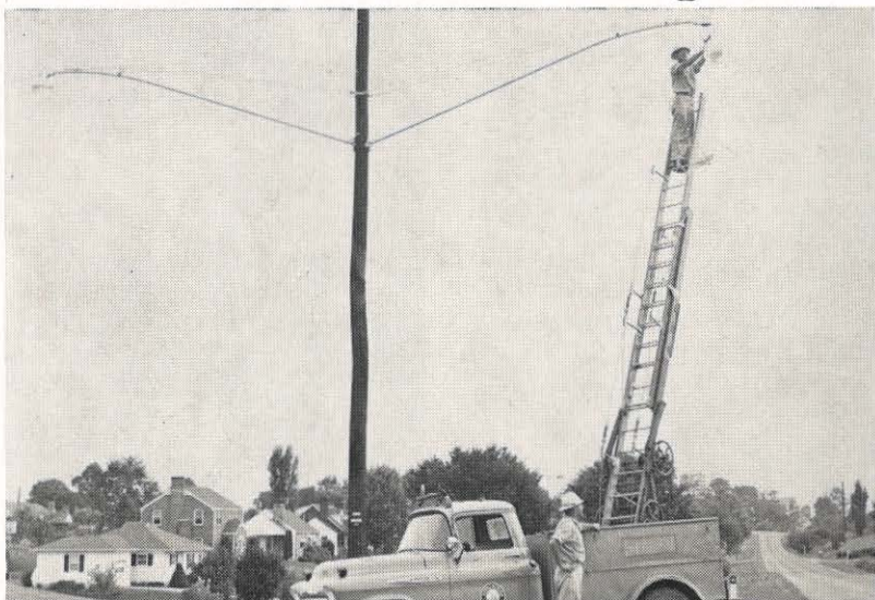
Area serviceman W. M. King and J. B. Nickols, meter serviceman, work on new street lights in a recently annexed section of Pulaski. The lights in this section were mounted on upsweep arms to effectively serve each lane of the divided highway.
