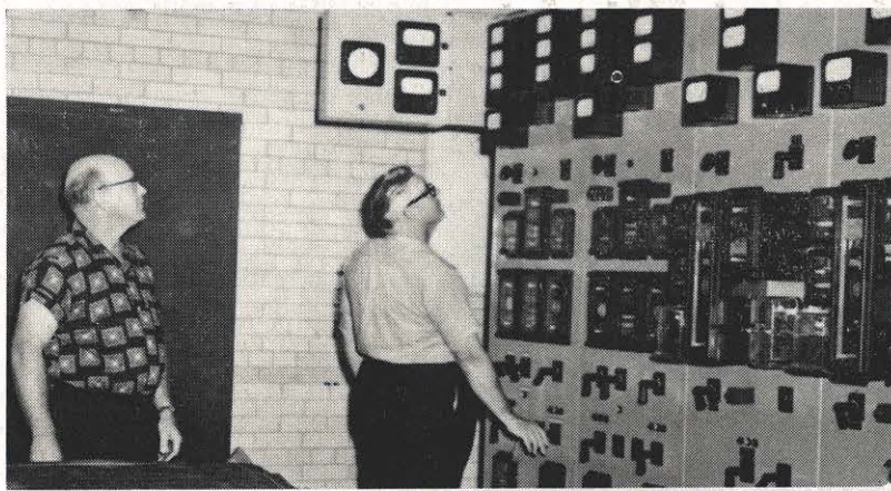
Lindsey B. Ferguson, regional chief dispatcher, throws a switch in the Philip Sporn station control room putting the new breaker-and-one-half system in Bay No. 5 into operation. Kermitt Ford, assistant regional chief dispatcher, watches.
