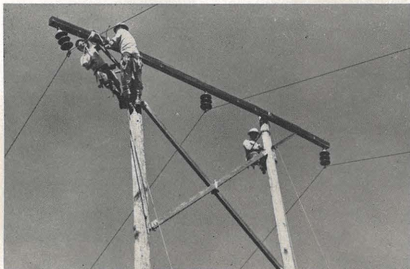
The co-ordination and planning of line maintenance work have become routine for our companies. Here, from left, linemen Earl Bellamy, Ira Smith and Auburn Helvey, Pikeville district, replace a cross-arm on a 46-kv line.
