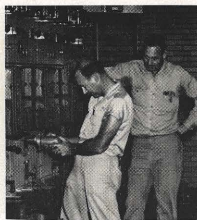
Lewis Chittum and C. E. Martin, system station switchboard branch, install new relay panels in the Sprigg station. The work, which enabled the station to handle the Clinch River plant load, took about 12 weeks.
