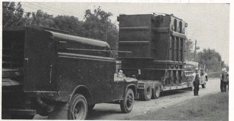
The 62½-ton transformer for Reedy Creek station near Kingsport was more than this tractor could handle. The tractor stalled on this slight grade, and two additional trucks were required to help complete the 5-mile trip to the new installation. This 60,000-kva transformer is the largest in the Kingsport area.
