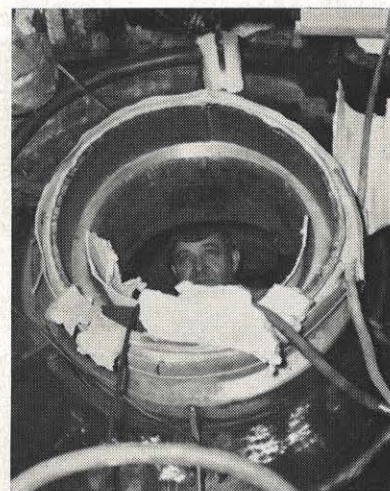
A worker peers through a boiler drum head being repaired after it developed a crack. The drum head is encased in a heating unit which was necessary to raise the temperature to 300 degrees for welding.
