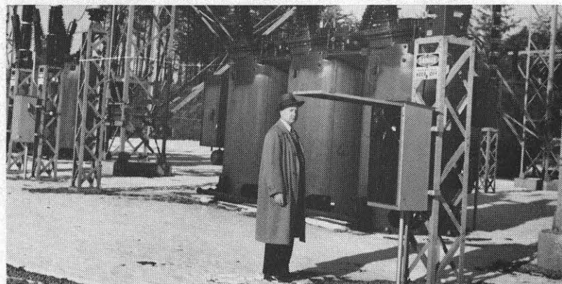
R. A. Armistead, Roanoke district line and station supervisor, pauses in his check of the new 20,000-kva Blaine station. The 138/13.2-kv structure serves the Thompson Products plant in Franklin County. It was placed in service in late November. The station has two 10,000-kva transformers.
