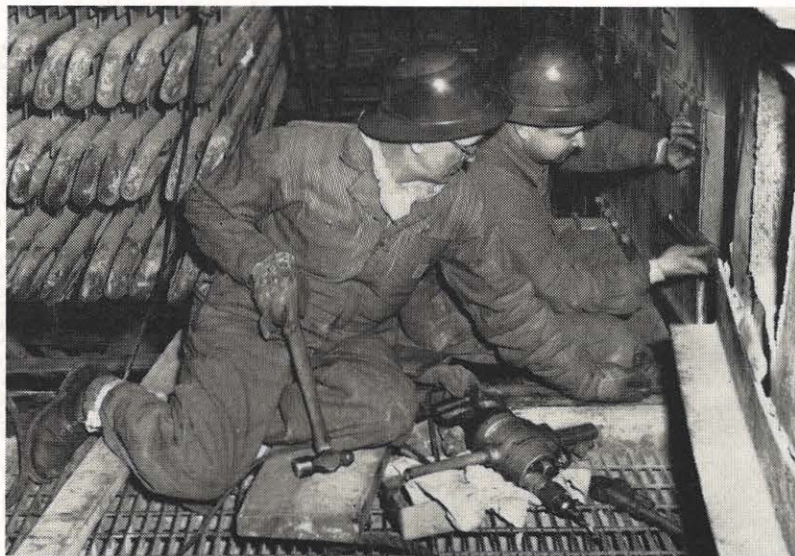
For the first time since 1954, Unit 5 at Glen Lyn plant has been removed for a six-week major overhaul. Here, R. B. McKenzie and E. W. DeHart, maintenance employees, prepare to remove economizer tubes in the No. 51 boiler for repairs. The main purpose of the overhaul is to retube the condenser, check wells and repair main steam lines, inspect control and stop valves on turbine, repair drum nozzle valve in boilers and many smaller jobs.
