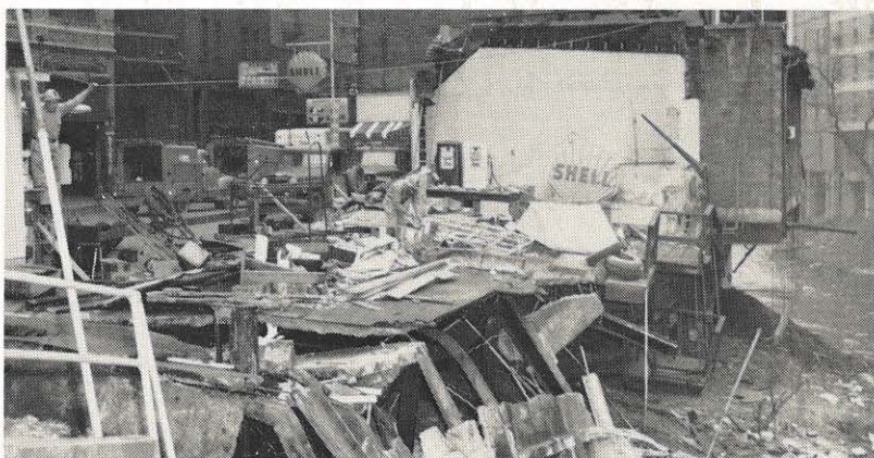
Three Welch meter servicemen work on the service wires in the wreckage left when steel supports under a gasoline station collapsed in Welch. Those working are Guy Albertson, James W. Nunnery and Charles Taylor.
