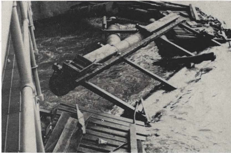
With the intruding barge out of the way, this is the repair task that awaited maintenance men at Marmet. This used to be the log boom.
