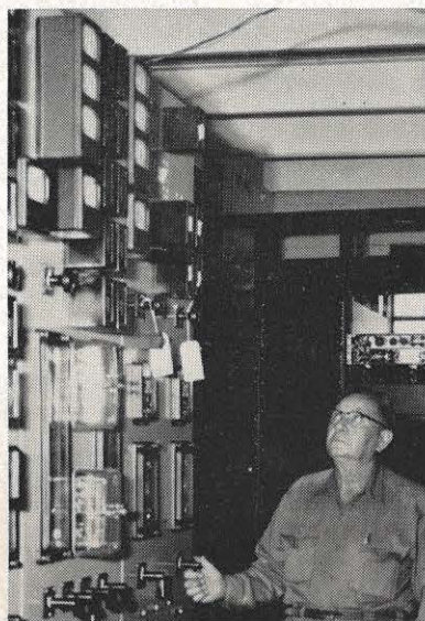
Checking the control panel for the Elk Mountain oil circuit breaker at Holston station is W. M. Childers, system station operator. The equipment is part of a new interconnection between Appalachian and Carolina Power & Light Company.
