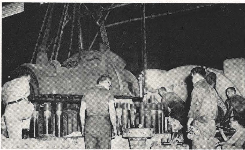
Shown as the inner shell of the high pressure turbine is being lifted for inspection of the rotor at Kanawha River plant are several employees. The work went on during an outage of Unit 1 at the plant. From left are: Amos Workman, W. A. Mitchell, who is a General Electric service engineer, William Ostrom, J. B. Caruthers, A. F. Hanning, J. R. Bostic, F. W. Holdren and G. E. LeMasters. Included in the work were the inspection of and necessary repairs to the high and low pressure turbines, sonic testing of the generator fields and repairs to the boiler superheater and reheater.
