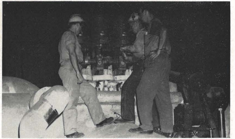
During an outage last month at Clinch River plant, these men worked on the control valves on Unit 1 turbine generator. They are from left: Lloyd McFarland, maintenance helper; W. H. Hall, maintenance man, and T. E. Peay, maintenance foreman.
