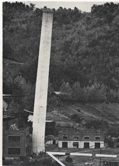
Flames licking greedily at its base, the stack at Hazard plant begins its fall. The broken line denotes the path the stack was supposed to take to the ground; the solid line shows the path it actually took.
