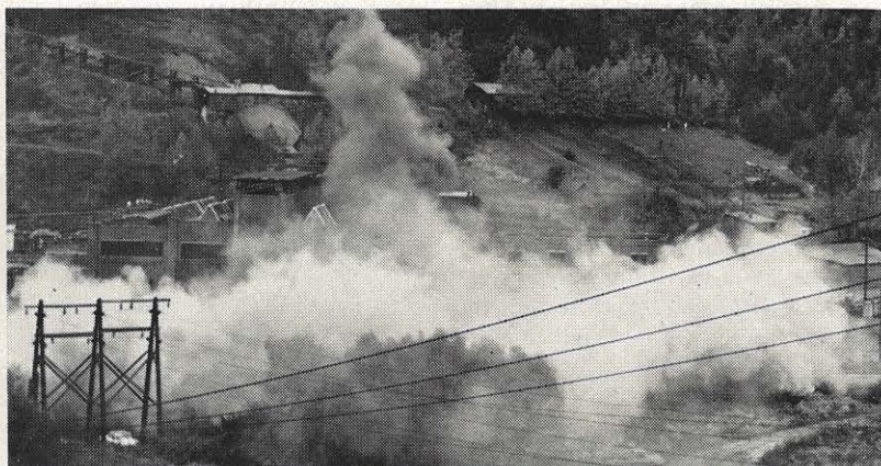
Dust and soot rise in the air as the stack crashes to the ground.
