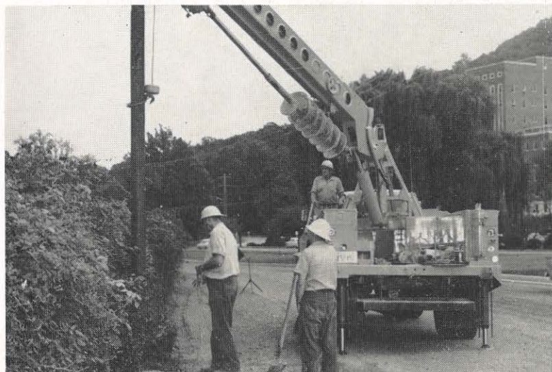
Working with the new equipment are, from left: R. D. Turner, foreman J. H. Witt and S. R. Ferguson. In this picture, the pole-setter is in action, the digger pulled up out of the way.
