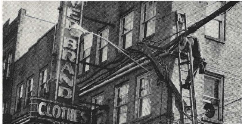
Aluminum conduits have alleviated a condition in Welch's main street. Here, M. K. Spraker, working foreman, on the ladder, is stringing power lines for the street in the conduit. This enabled the combining of several lines in the conduit, eliminating many wires and brackets that extended out over the street. The conduits themselves are new, and the company has received many favorable comments on the work.
