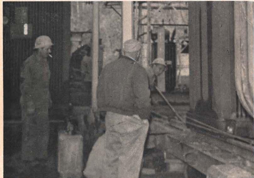
Hazard district men continue work at the Hazard plant. Here Fred Barnett, Edgar Pigman and Ernest Pennington are removing three 1,667 kva transformers, scheduled to be replaced by 2,500 kva transformers in the switchyard. They will serve a 5,000 kva condenser in the plant building.
