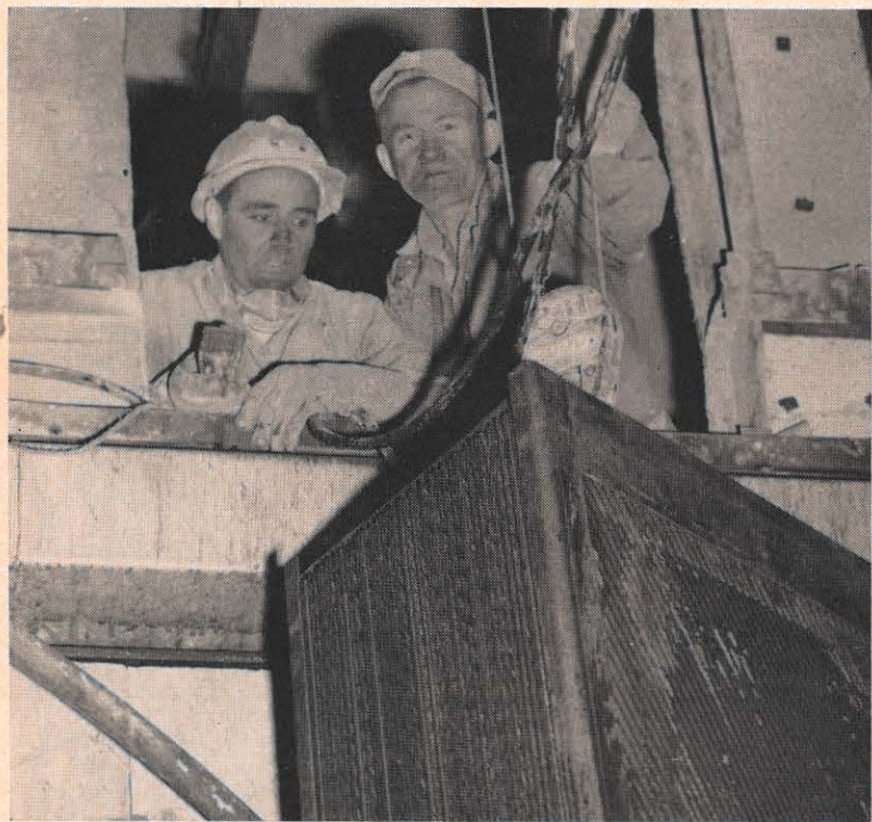
A new technique to clean the air preheater baskets was worked out during a recent outage at Clinch River Unit No. 1. All 720 baskets were removed, soaked in acid solution, and then flushed with clear water at 250-lbs. per square inch.
