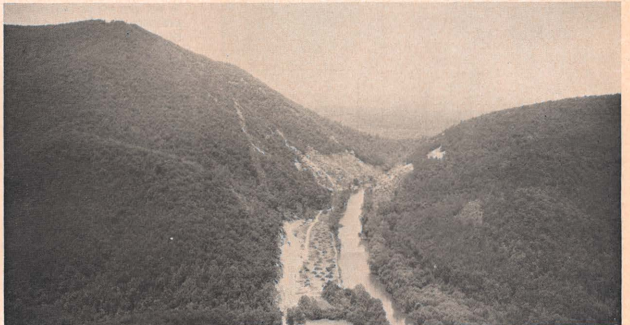
This photo is looking upstream at Smith Mountain Gap, where a large amount of work is being done on the upper dam in the Smith Mountain Combination Hydro-electric Project. Most of the work is being concentrated on the north, or right, side as it appears here in this photo taken a few weeks ago.
