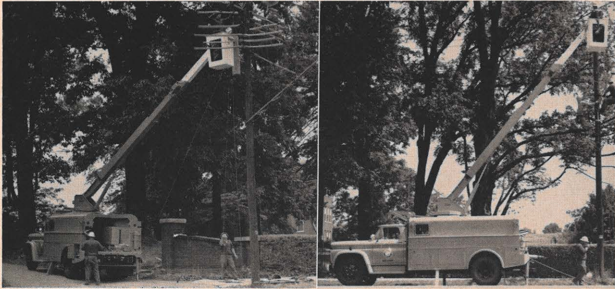
Appalachian's versatile new truck gets its first on-the-job workout. At left, work on a distribution line is being done by the Washington County line crew with the invaluable aid of the truck and its bucket. R. E. Crusenberry is in the bucket, covering the line. Assisting him in
