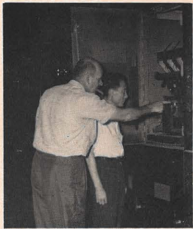
J. A. Moore, Cabin Creek plant manager, shows Chung Sun a 2300-volt air circuit breaker in the course of Mr. Sun's week-long visit at the plant.
