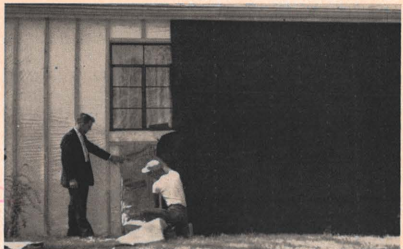
This photograph is practically a cross-section showing how insulation was applied to the outside of a house in Charleston. Behind H. K. Shabdue, standing at left, the house is covered with polyethylene with furring strips nailed over the plastic. Under the window a contractor's man is installing Fiberglas insulation, and to the right, the house is covered with building felt. A stucco finish went over that to complete the job.
