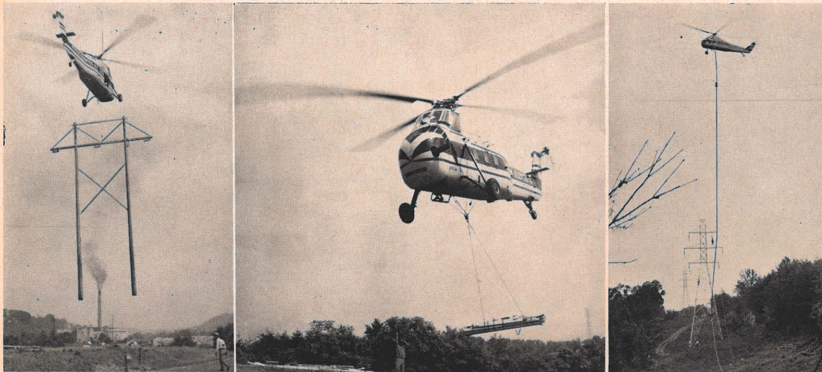
Three major phases of work involving the helicopter are pictured here. At left, the helicopter is leaving a marshalling yard adjacent to the Owens-Illinois Company plant at Big Island with an H-frame structure. Wood poles are being transported by the helicopter to their sites, where they are being
