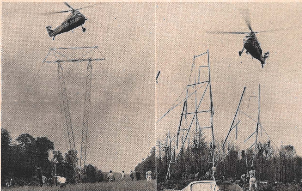
As further tests of the capabilities of the helicopter in line work, these two experiments were successfully tried during construction of Appalachian's two new lines. At left, an entire structure, made of aluminum, was picked up at a marshalling yard by the helicopter, borne to its site and placed. Here, crews on the ground tie in the
