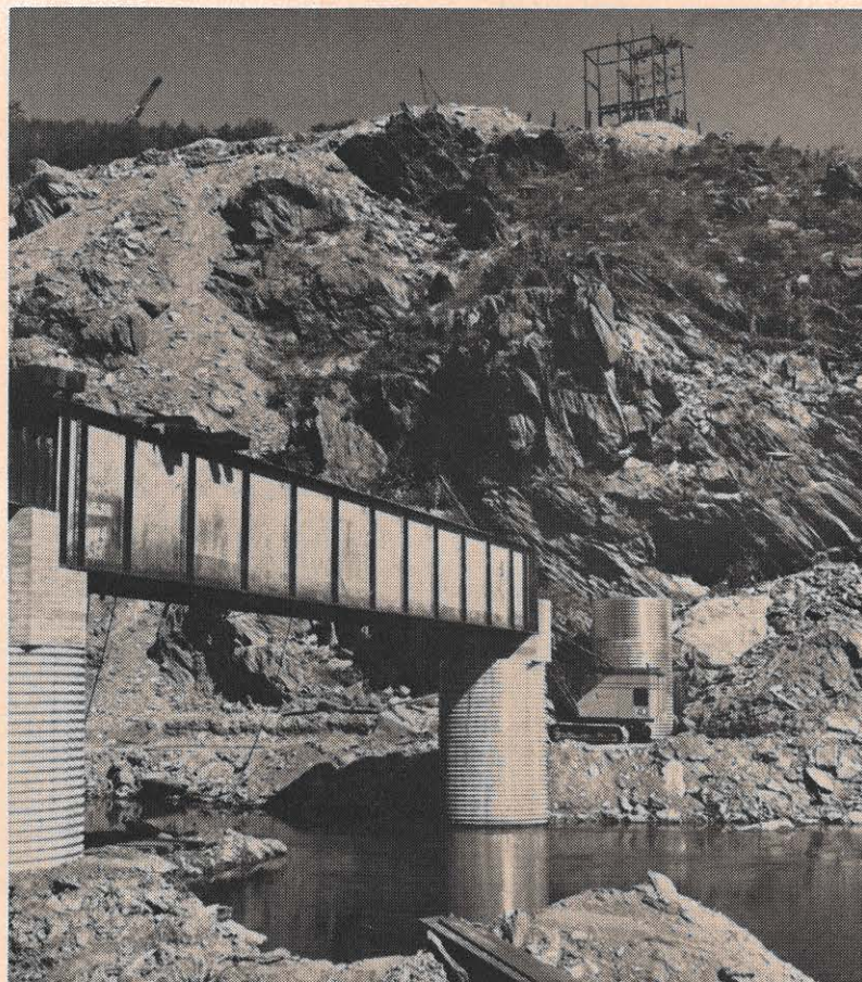
Progress is being made on the construction of this bridge across the Roanoke River at the Smith Mountain Dam site. The bridge will be used to transport material to the concrete plant. Photo courtesy Times-World Corp.
