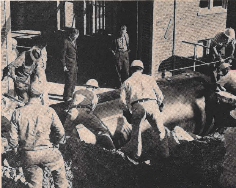
The Bluefield line crew has to be jacks-of-all-trades, because there is always something different to do. The 1,000-gallon gasoline tank at the Bluefield garage developed a leak, and the crew was called on to replace it. In three days, the old one was dug up; a new and larger one installed, the hole filled in and the surface paved over. Here the crew lowers the new tank in place.
