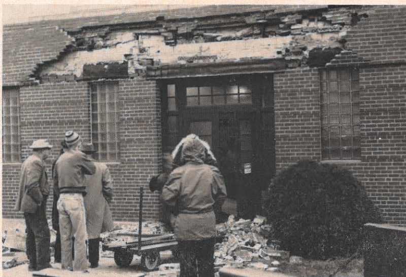
Kingsport Utilities men survey the damage caused by an explosion at the company's Cumberland station December 21. The mishap knocked out electric service in downtown Kingsport for a few hours.
