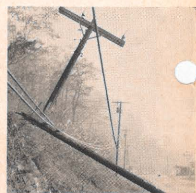
This pole in the Logan district stayed like this for six hours after it was snapped by a speeding car. It carried a four-wire 12,000-volt circuit, a television cable, and two trunk-like telephone cables. Service was interrupted only momentarily.
