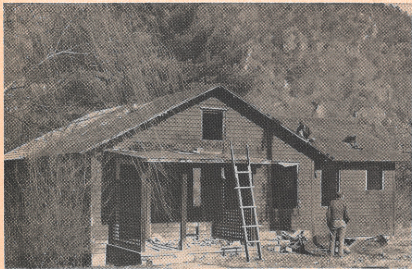
End of an era: workers begin dismantling a company cottage that stood in Buck camp for nearly a half-century.
