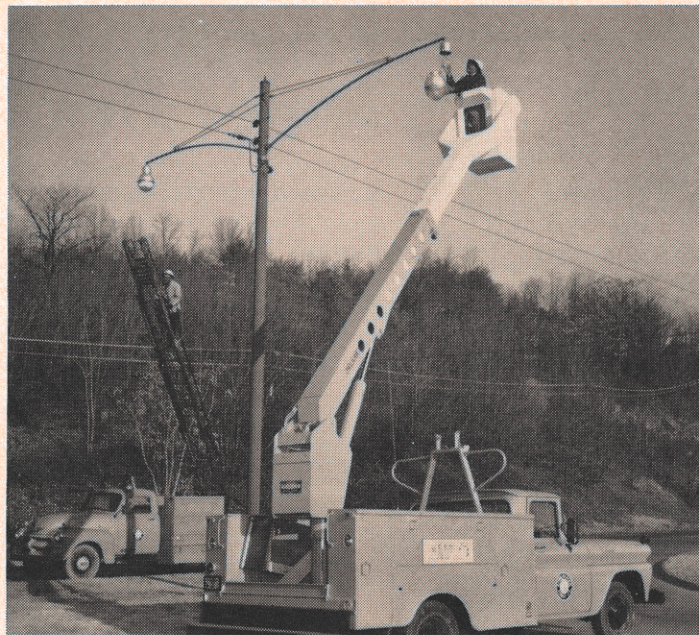
A demonstration of one of the major advantages of Roanoke's new truck—speed—is shown at left. While A. S. Pullen is already replacing a street light using the new truck and its hydraulic boom and fiberglass bucket, J. M. Brown at left, using the old ladder truck, is still not
