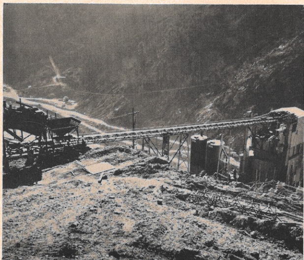
The concrete mixing plant at Smith Mountain seems to be perched precariously on the edge of the mountain side; but there's room below it for a railway to carry buckets from the plant to the cableway, which in turn will carry the concrete out over the dam. The conveyor belt here
