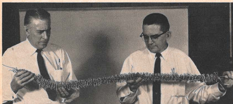
During a recent windstorm in Huntington a tree fell on a 4-kv line, and broke the No. 2ACSR conductor. The result was a strange compression pattern, examined here by Paul Harlan, left, line supervisor, and Fred Schwartz, district superintendent.
