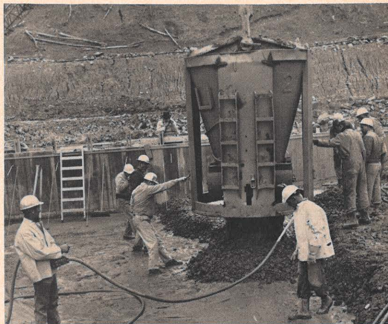
Four cubic yards of concrete are released from the bucket, part of the approximately 850 cubic yards poured in this first concrete work at either dam.
