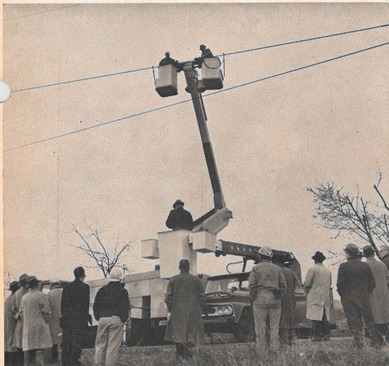
Before a rapt audience of company personnel and a scattering of newsmen, J. B. Doss, general foreman, and R. J. Fisher, foreman, of the system transmission line department, demonstrated the revolutionary "bare hands" maintenance technique in Roanoke last month. The idea, based on the principle that current does not flow when there is no difference in voltage between two points, was developed into workable practice by American Electric Power Service Corporation engineers, and announced last fall by Philip Sporn, AEP president. Harold Rorden, AEP high voltage practices engineer, was in charge of the demonstration, designed to determine the method's merits in the various terrains and under various conditions existing in the company area.
