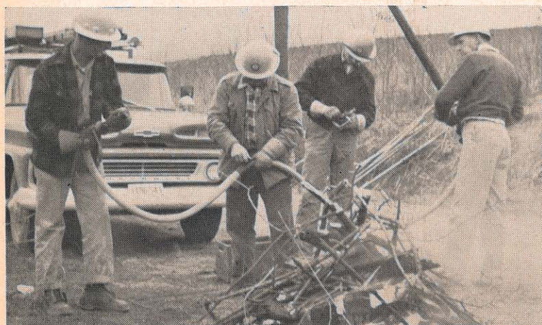
This photo illustrates one of the conditions our people work under to keep our service to customers at its dependable best. This Pearisburg line crew is working in freezing April weather to move a line, without interruption to service. They have made one concession to the cold—they have built a fire, and staying by it to prepare a hot-line jumper so the line can be kept energized while crossarms and hardware are moved from the old pole to the new one, side by side. In the picture are, from left: Willie B. Rasnake, David R. Mann, Clifford L. Dunigan and Harry B. Boyd, all linemen. Pearisburg is in the Bluefield district.
