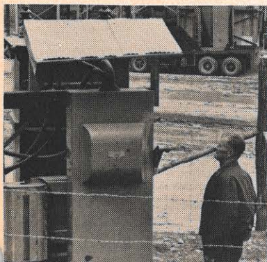
At Leesville, Harry Snead, chief of electrical section, handles all temporary power, including this construction transformer bank, which he is shown checking. In the background can be seen a truck at the concrete batching plant.
