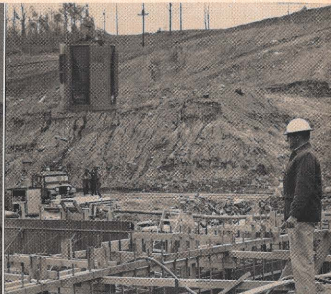
Homer Martin, engineer in charge at the Leesville Dam, watches as a four-cubic-yard bucket of concrete swings into the spillway section, where the first concrete in the two-dam project was poured in April. This picture is looking south, and one side of the dam will be built into the hill back of Mr. Martin. Appalachian and construction company offices at the site of the smaller of the two dams are out of view on top of the hill.
