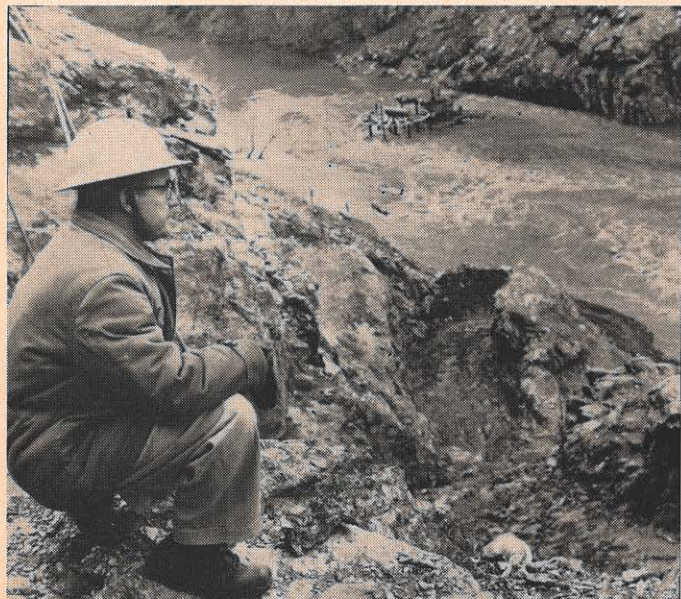
George Bentley, structural engineer at Smith Mountain Dam, pauses on the south side of the mountain as the Roanoke River goes by below him. The cut in the rocks leading to the river is for the keyways. Mr. Bentley is supervising rock cleaning and foundation preparation in this area. In the river is the start of a piling cell, part of the scheme that, when completed, will divert the river for construction.
