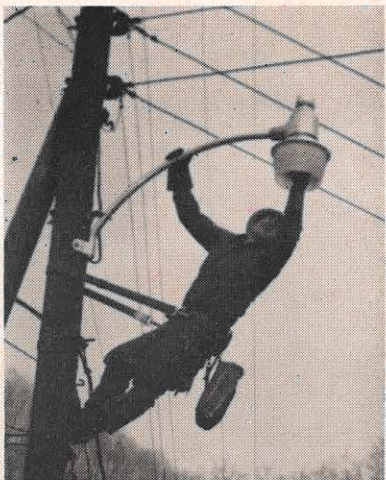
J. W. Nunnery, Welch meter serviceman, puts the final touches on the installation of a 7000-lumen dusk-to-dawn light. This one was received in the storeroom at 2.30 p.m. and installed at 3 p.m.
