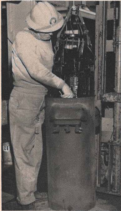
J. R. Hughes, stationman, removes the core and coils from an old transformer for inspection, cleaning and reconditioning in the Johnsons Lane repair shop.
