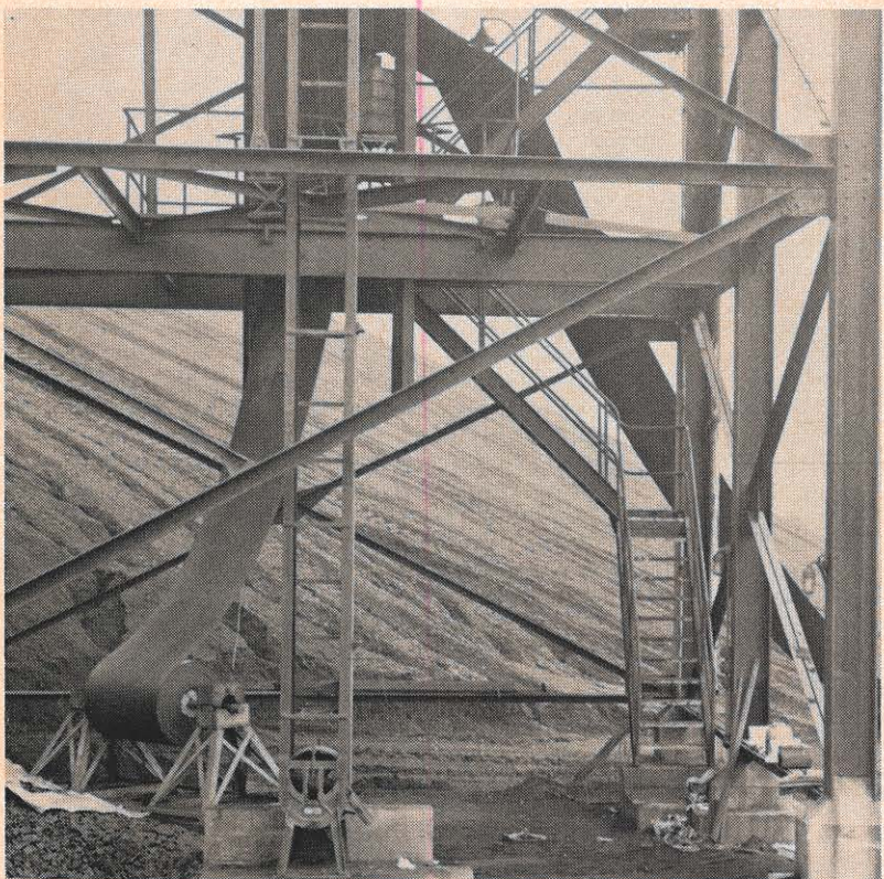
The original belt on Kanawha River plant's No. 2 conveyor was replaced last month in an interesting fashion. The old belt was cut, and the end of the new belt attached to it. The other end of the old belt was attached to a truck; as the truck was driven away, the action wound up the old belt and threaded the new one in place.
