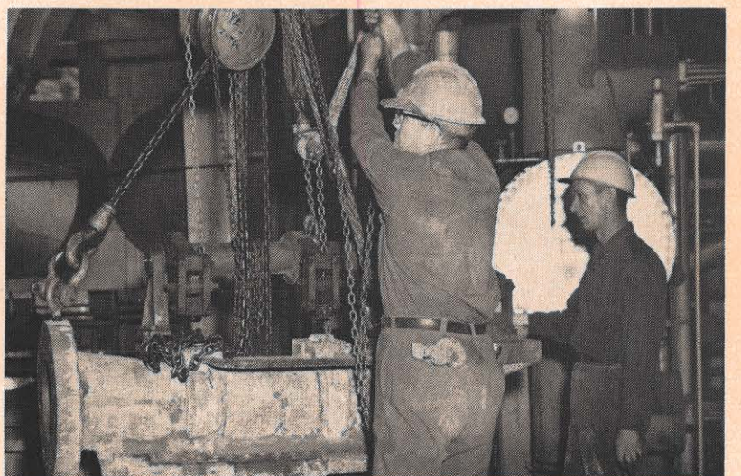
Conrad Powers, left, and Lovell McDonald, master maintenance men, are working at Clinch River plant during removal of Unit 2's boiler feed pump steam chest. The unit was out from July 1 to July 16 to rebuild the ash hopper following redesign. For three days during that period, Unit 1 was also out for maintenance and repair.
