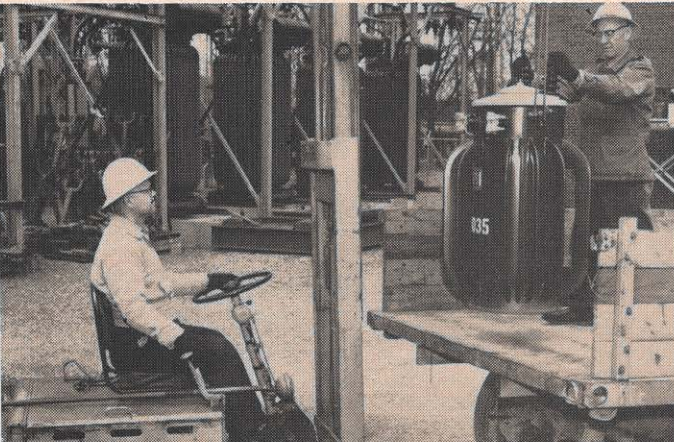
A new transformer from the Johnsons Lane storage yard, where it was checked out after manufacturer's delivery, is hoisted on a truck. H. H. Purdue and Frank C. Lake, stationmen, are doing the work.
