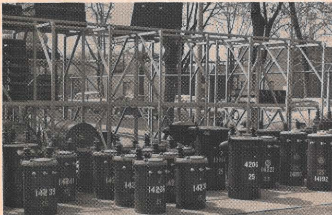
Rows of distribution transformers, invaluable equipment in getting dependable, low cost electric power to our customers, await their turn for installation at the yard at the Huntington storeroom.
