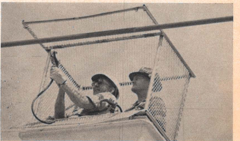
For the first time, an Appalachian 345,000 volt line has been worked with bare hands while it was energized. It happened at Kanawha River plant on the Kanawha-Spohn line, on which surge tests were being run. Here, L. H. White of Ohio Power is connecting a clamp to energize the wire mesh in the Fiberglas bucket to the same voltage as the line, while Harold Rorden, high voltage practices engineer of the AEP Service Corporation, observes. Mr. Rorden developed the basic idea and has supervised the research and testing on barehands work.
