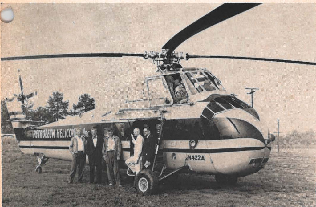
When the AEP System in 1960 carried out its first transmission line construction by the use of helicopters, Mr. Sporn was on hand to inspect the job personally. Here, Sporn (in light suit), alights from helicopter at staging area in Virginia. Other System officials in photo include H. A. Kammer (in bow tie) and R. E. Hodges (right).
