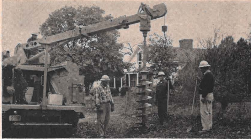
Roanoke district has recently placed in service this truck, designed by Appalachian, that makes installation of poles quicker and easier. Using hydraulic controls, the truck does the entire job of digging the hole and setting the pole. C. T. Rader, truck driver-groundman; R. D. Turner, working foreman; H. F. Carter, lineman; and J. C. Thomas, groundman, are the crew.
