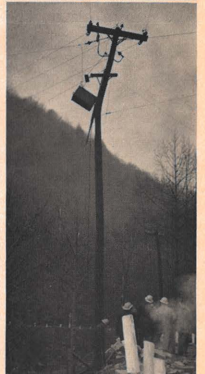
In the course of highway widening work near Welch, a dynamite blast scattered rocks in all directions, one of them smashing this service pole and breaking it as shown here. By a rarity no outage resulted from this mishap, even though some equipment was damaged.
