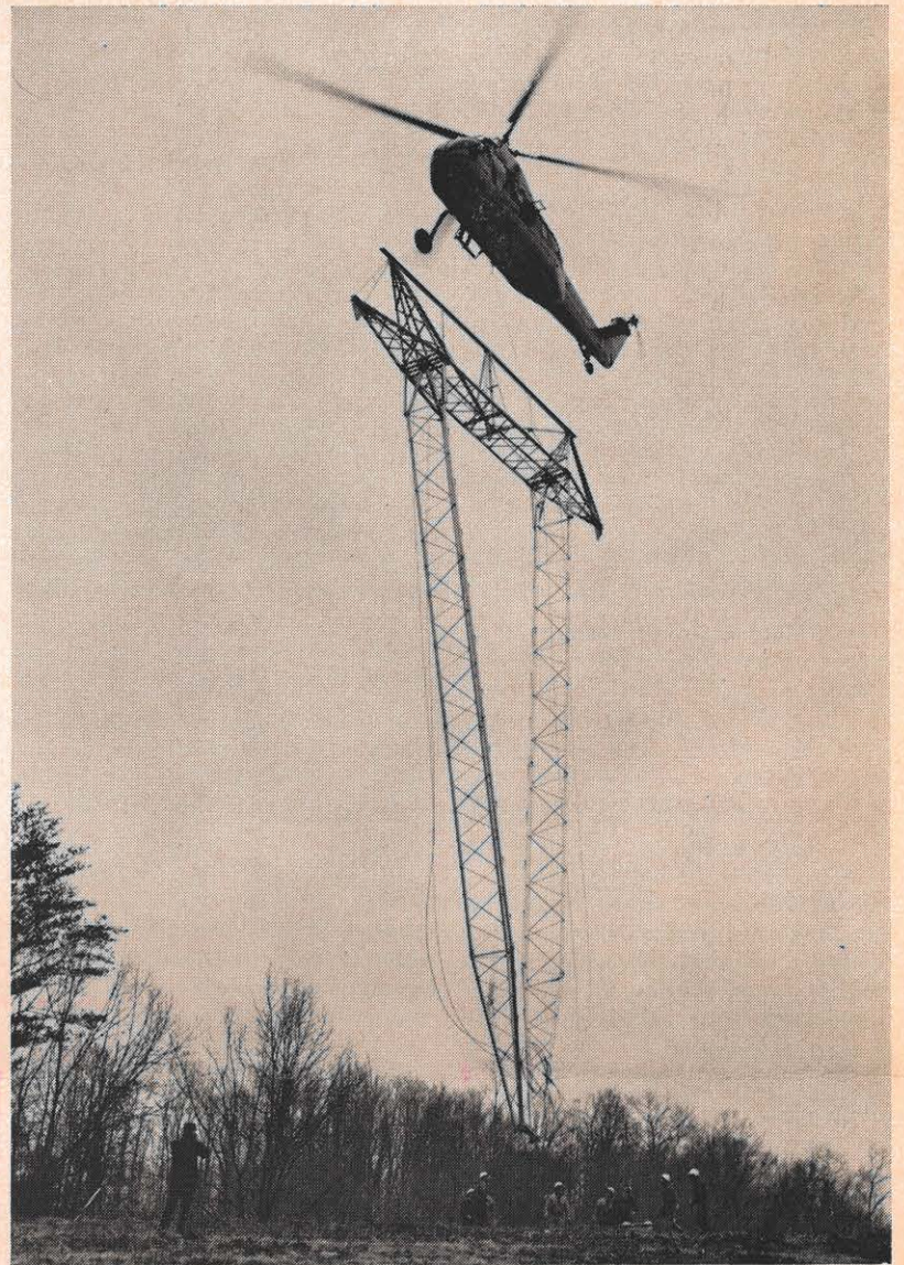
After picking up the V-shaped aluminum tower at a marshalling yard and transporting it to its site, the helicopter brings it into position. The ground crew is guiding the tower to its central anchor.
