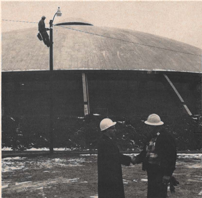
W. C. McMahan, Beckley district manager, congratulates E. A. Berginnis, line foreman, on the 1,000th Dusk-To-Dawn light installation in the district. K. K. Keatley, lineman, is making adjustments on the last of six units installed at Beckley's new Armory and Civic Center.
