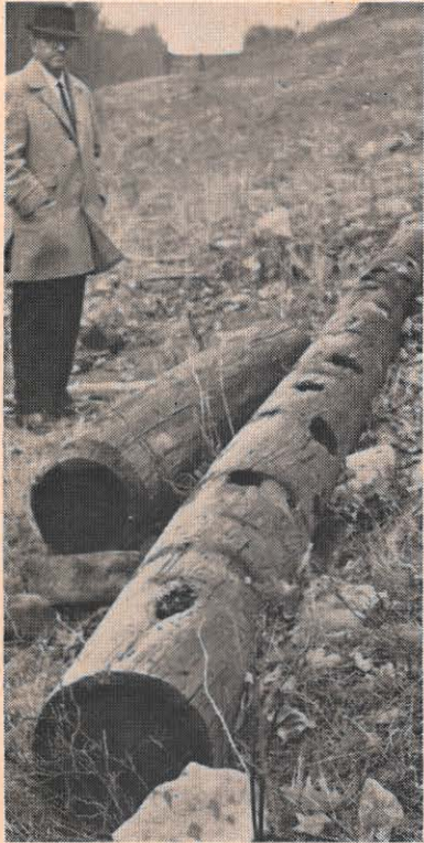
Woodpeckers can peck a lot of wood. M. R. Callaway, Bluefield district right-of-way agent, ruefully totals up the damage done to this 40-foot pine pole: 37 holes, averaging three inches in diameter and two to three inches in depth.
