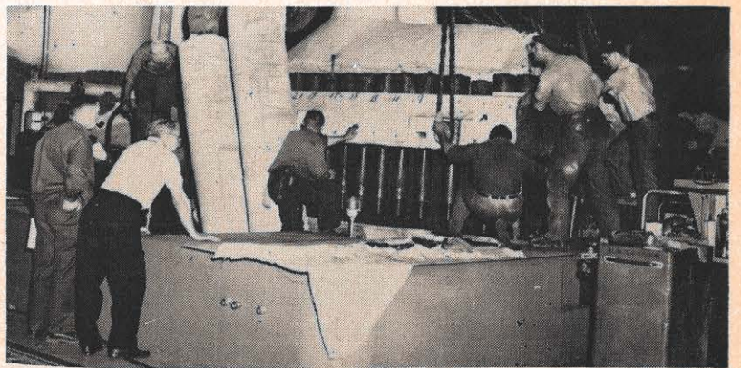
Work on Unit 5 during its 7-week outage at Philip Sporn plant was completed on schedule. Here, Ralph Warner, plant engineer, and Bill Mitchell, General Electric, watch as plant employees assemble the high pressure turbine shell. Both high and low pressure generators were rewound by GE, and several other repairs, replacements and inspections of the unit were made while it was down.
