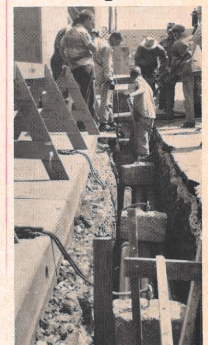
Electric service in some portions of downtown Bluefield are going underground. Duct work is half completed and will carry three circuits. The work is being done on portions of Bland, Ramsey, Scott and Federal Streets. There will be 1,300 feet of primary cable, carrying 12,000 volts, a transformer in a vault, three man-holes and two pull boxes. Work is to be finished by mid-August.
