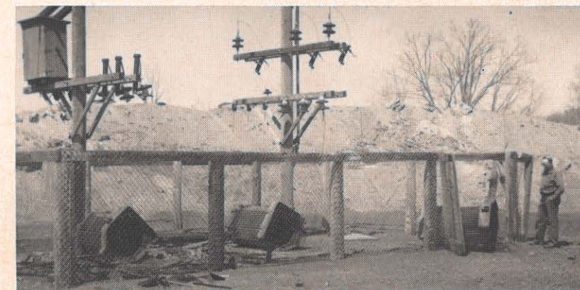
Ralph Slade examines what is left after thieves hit this station, making away with much material and hardware.
