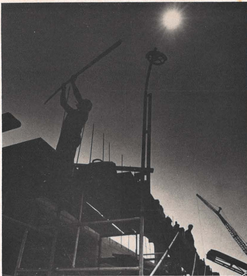
Symbolizing industrial activity in the Roanoke district of Appalachian is this "Roanoke World-News" picture of construction at the Sealtest plant in the Blue Ridge Park for Industry.
