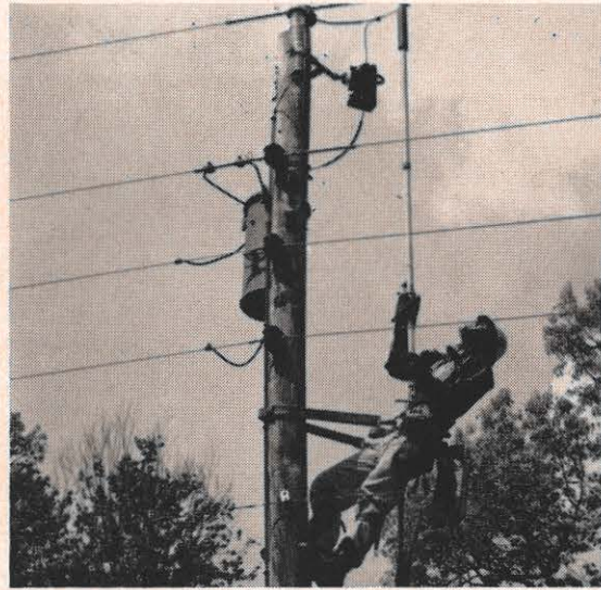
These three pictures catch Mr. Shrader in a variety of tasks performed during the course of a single day recently. At left he replaces line connections
