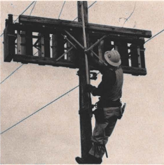
on a transformer pole to clear up radio trouble experienced by a customer; in the middle picture he climbs a pole again to replace a fuse on a
