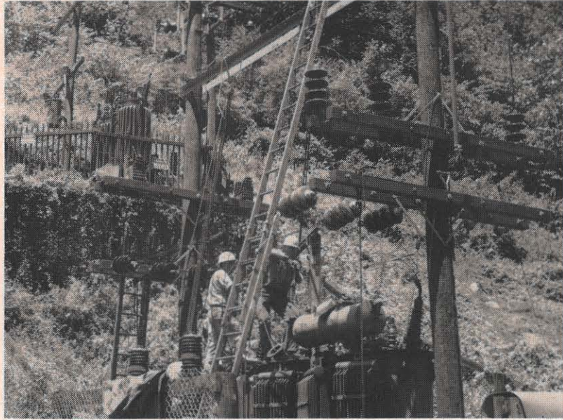
The miners' vacation every July gives Appalachian crews in the coal country a chance to catch up station maintenance, often the only chance of the year. Electric service still must be available to other customers, however, and to solve the problem, temporary stations are put into service. One of the two used in the Welch district this year is shown here.
