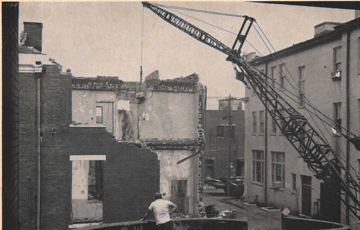
Right in step with Charleston's drive to clean up the capital city is the Charleston office of Appalachian. A persuasive one-ton boom brought down the old red brick building back of the office to make way for a
