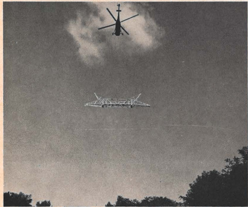
One hot day on Catawba mountain, the helicopter was silhouetted against a cloud while carrying the top part of a tower: the bridge, the arms, and the goat-heads. It was sometimes necessary to carry parts of towers to their sites to be reassembled. Later the helicopter would return to raise the tower in place.
