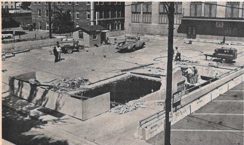
A gaping hole, one of several being cut in the former ramp, is evidence of work beginning on the addition to Appalachian's general office building in Roanoke.
