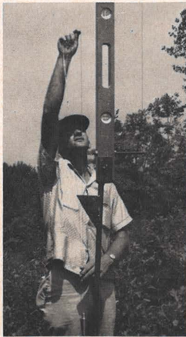
The foreman of a setting crew checks with a level and bob to make sure that the tower is level. By loosening and tightening guy wires, the crew is able to follow his instructions, and bring the tower erect.
