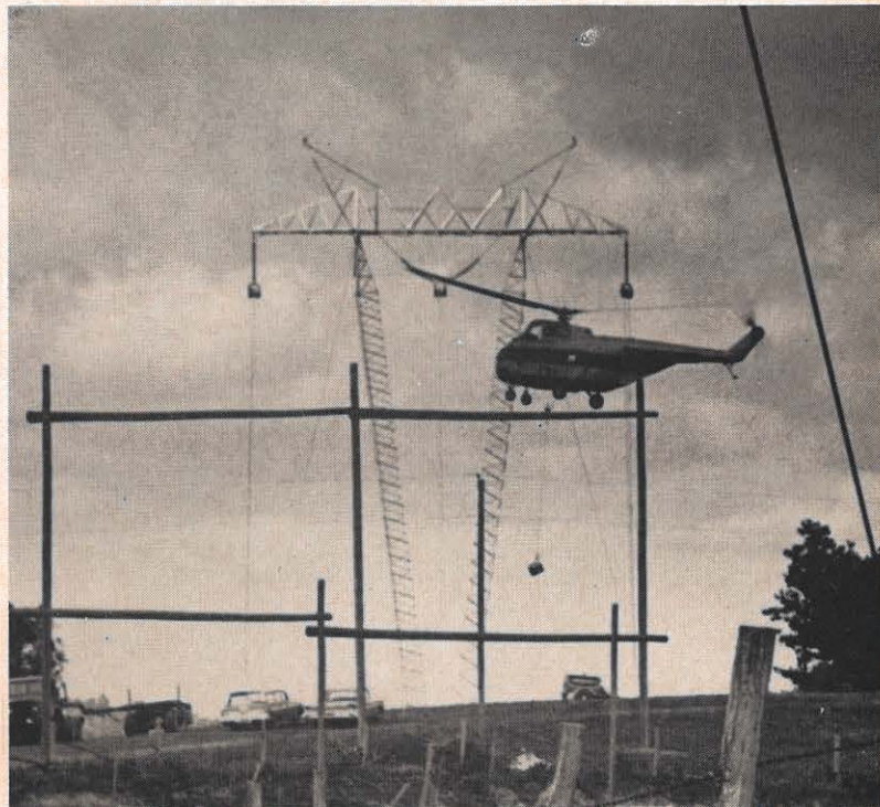
Erection of the towers was completed in August, and work began on stringing the conductor and ground wire. A helicopter was used on this job too, carrying the lead line for the conductor from tower to tower; the lead line is made fast to the conductor, which is then pulled through by winching.
