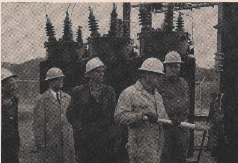
H. A. Hale has an interested audience as he energizes the new Roanoke Division 34.5/12-kv station at New Castle. Watching, from left, are: J. H. Mann, J. B. Whitmore, W. S. Shanks, and T. G. Reynolds. The new station strengthens service to the town of New Castle, near Roanoke, and the surrounding area.
