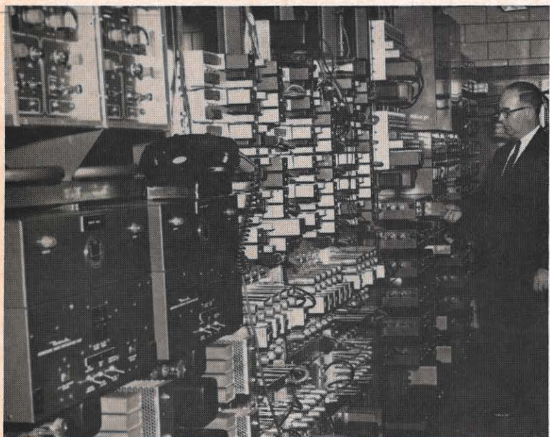
George M. Guill checks a portion of the microwave equipment in the microwave room atop the Roanoke office building. Equipment shown here handles both of Appalachian's microwave systems.
