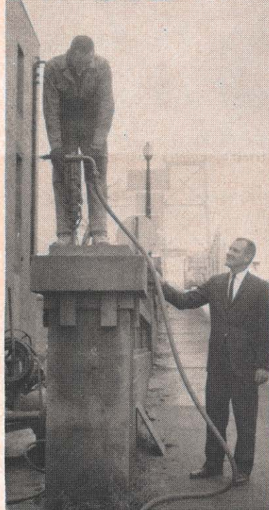
O. C. Hall, Point Pleasant district superintendent, and president of the Chamber of Commerce, watches with satisfaction as work begins on installing street lights...
