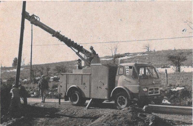
A new line truck was put into service at Abingdon at the first of the year, and features a hydraulic boom with an auger.
