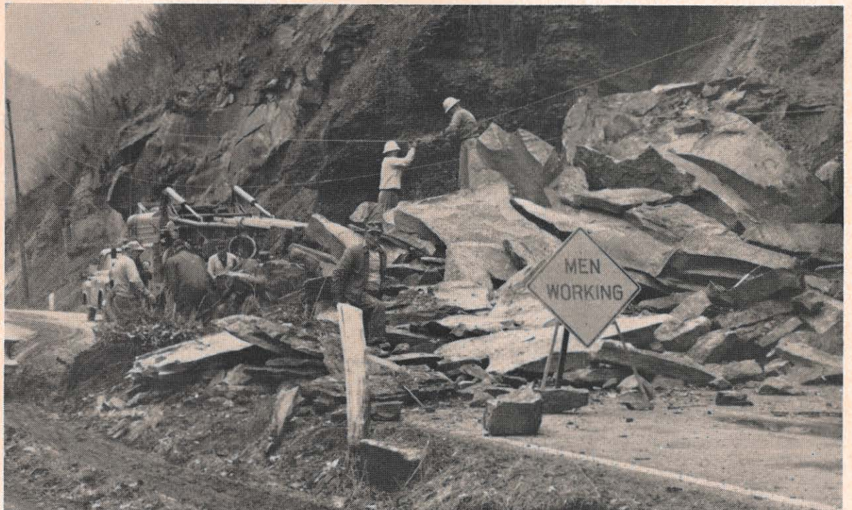
March came in with wind and rain around Charleston, and caused many rock slides like this one near Gauley Bridge. O. J. Hundley's crew from Montgomery repair sagging lines while state highway department men clear away the rock that blocked U. S. 119. The two men at the line are Mr. Hundley and Fred Dooley. (Photo courtesy Bronson McClung and the West Virginia Hillbilly.)
