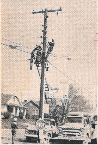
The first dusk-to-dawn light installed in Tazewell County, having served a noble purpose, now gives way to a 21,000 mercury vapor luminaire. The light was originally put up in Riverjack, which has recently been annexed by Tazewell. There are now about 395 dusk-to-dawns in Tazewell County and 1399 in the Bluefield district.
