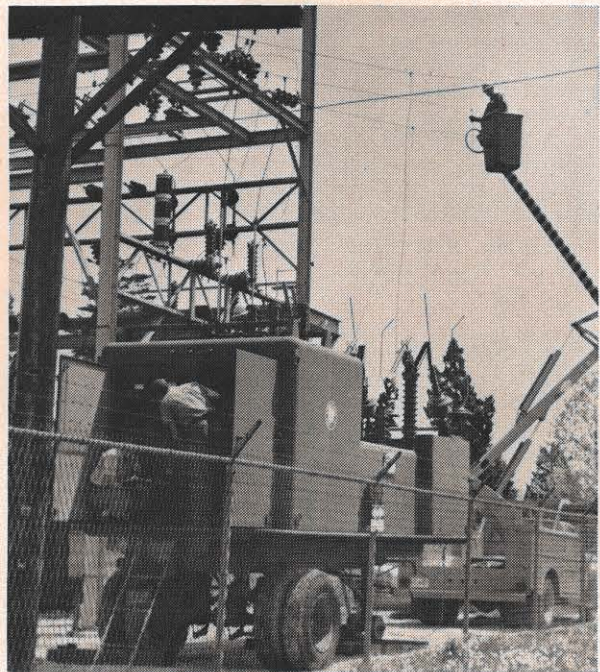
By using a 3,000 Kva 34.5/12 mobile substation, the Pulaski district station crew was able to work on the Lee-Hi station without interrupting service to Wytheville and parts of the surrounding area. The unit was moved in from Bluefield and connected with the help of an aerial bucket, and the job was done on a Sunday afternoon.
